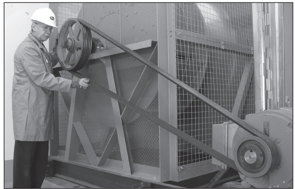
Carefully inspect all belts
